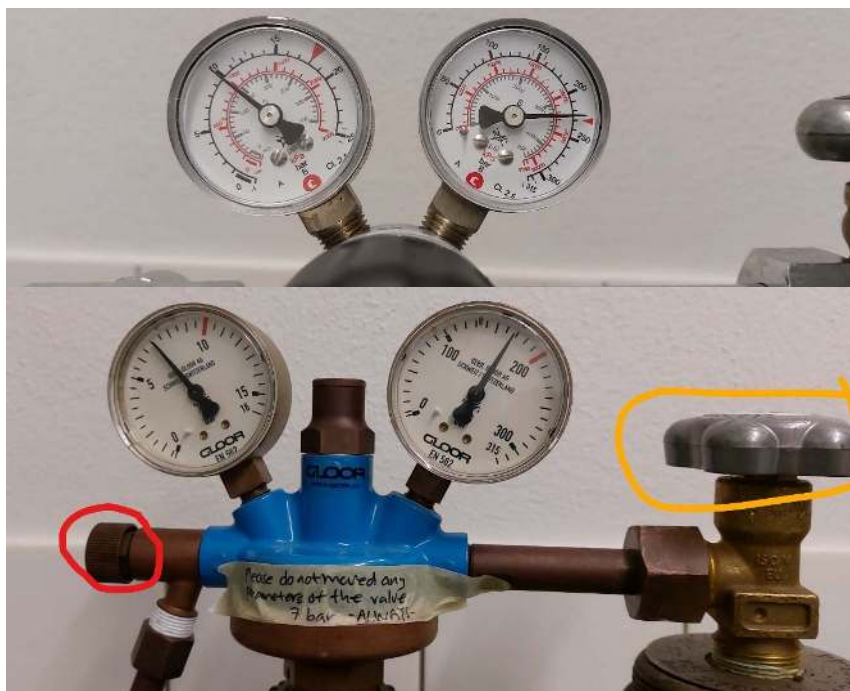
Figure 2. Nitrogen tank (top) and pressurize air (bottom) with correct settings. Yellow circles illustrated the main tank opening. Red circle in pressurized air need to be open always except when the tank need to be change.
