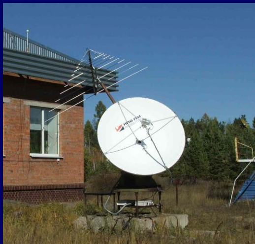
Antenna attached to dish
